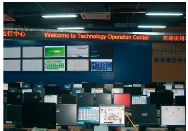
Technology operation center Beijing
